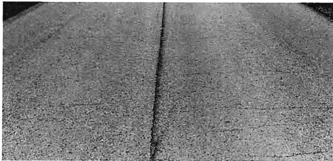
Centerline crack (still tight). ▶
