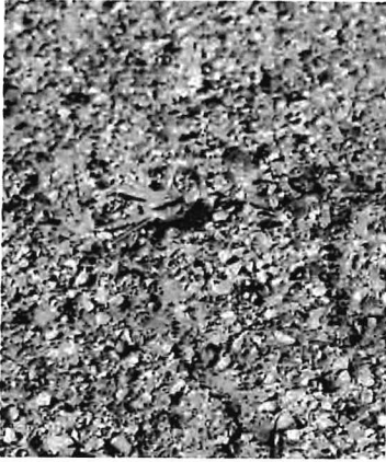
Severe raveling with ▼ extreme loss of aggregate.
