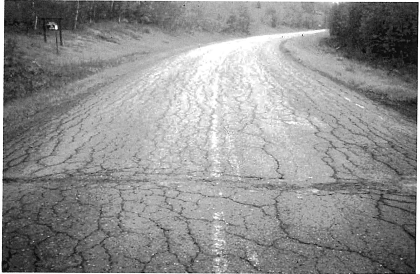
▶ Extensive alligator cracking. Pulverize and rebuild.
