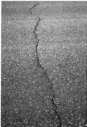
▲ Tight cracks less than 1/4" in width.
