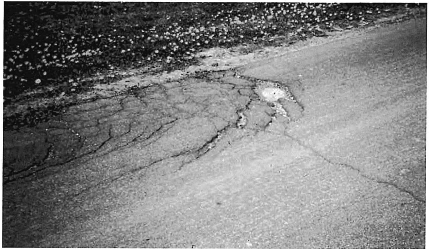
► Crescent-shaped cracks characteristic of slippage.
