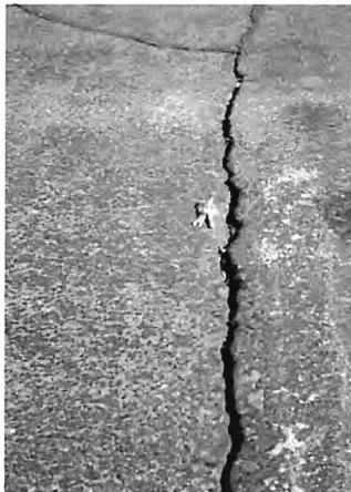
▲ Open crack – 1/2" or more in width.
