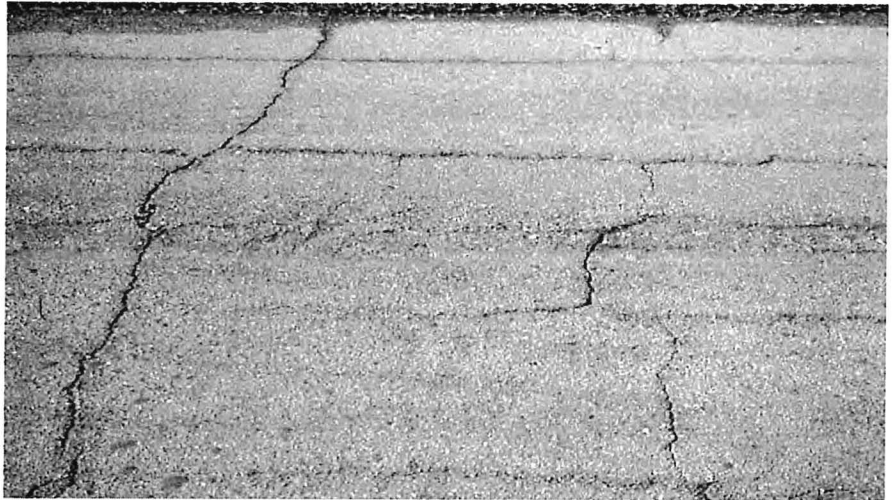
▼ Block cracking with open cracks.
