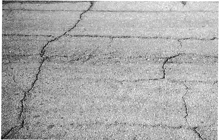
▶ Intermediate-size block cracking, 1'-5' across with open cracks.
