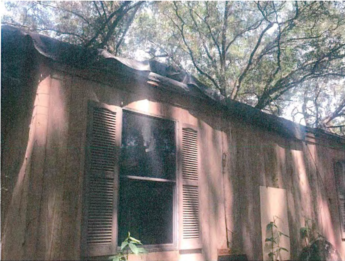
LEFT & SOUTH SIDE VIEW OF MOBILE HOME: ROOF TARPS COVERING DAMAGE
