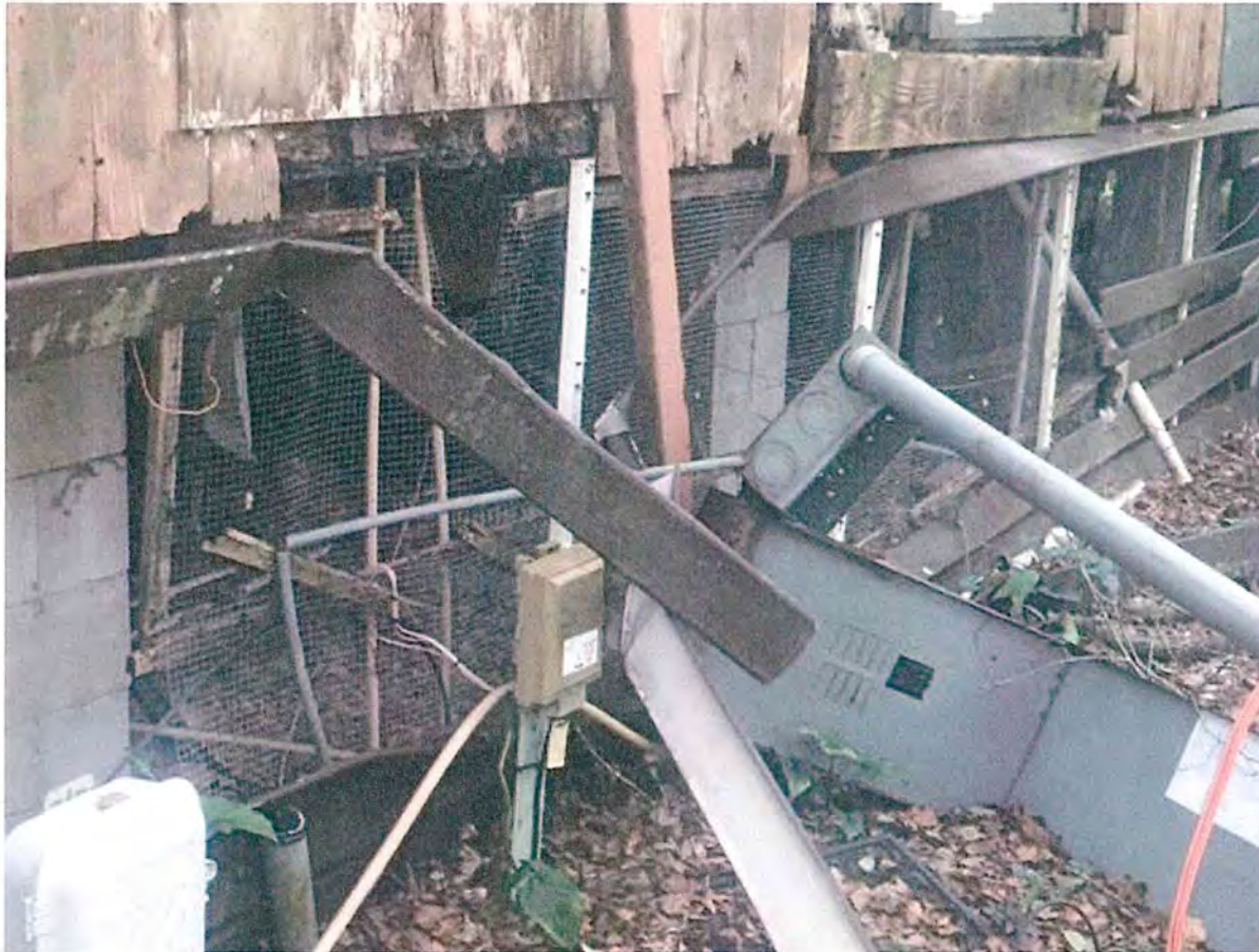
RIGHT & NORTH SIDE VIEW OF MOBILE HOME: ELECTRIC PANEL BOX REMOVED
