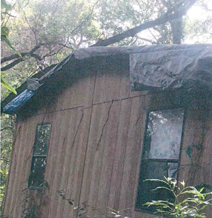
REAR & EAST SIDE VIEW OF MOBILE HOME: ROOF TARPS
