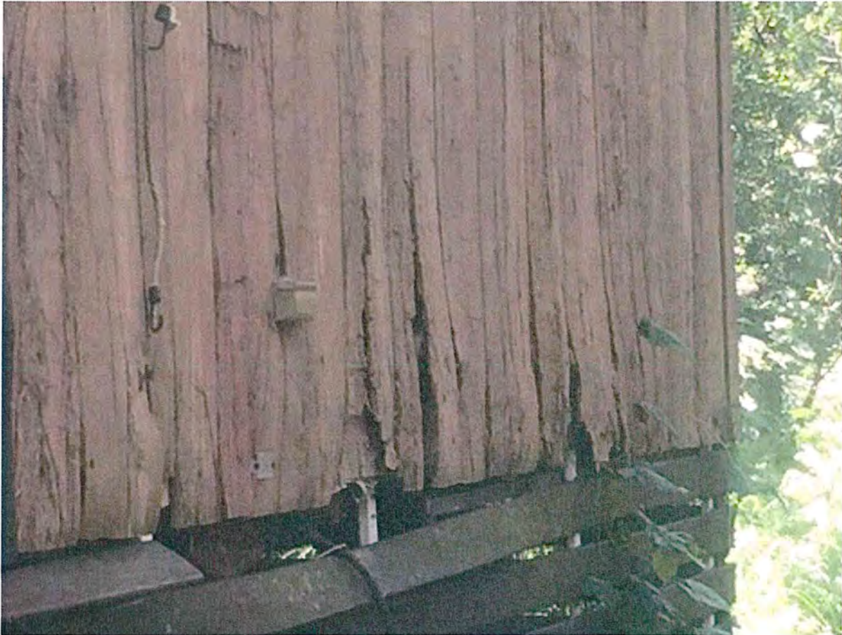
RIGHT & NORTH SIDE VIEW OF MOBILE HOME: NORTH WEST CORNER WALL AND SIDING ROT & DECAY
