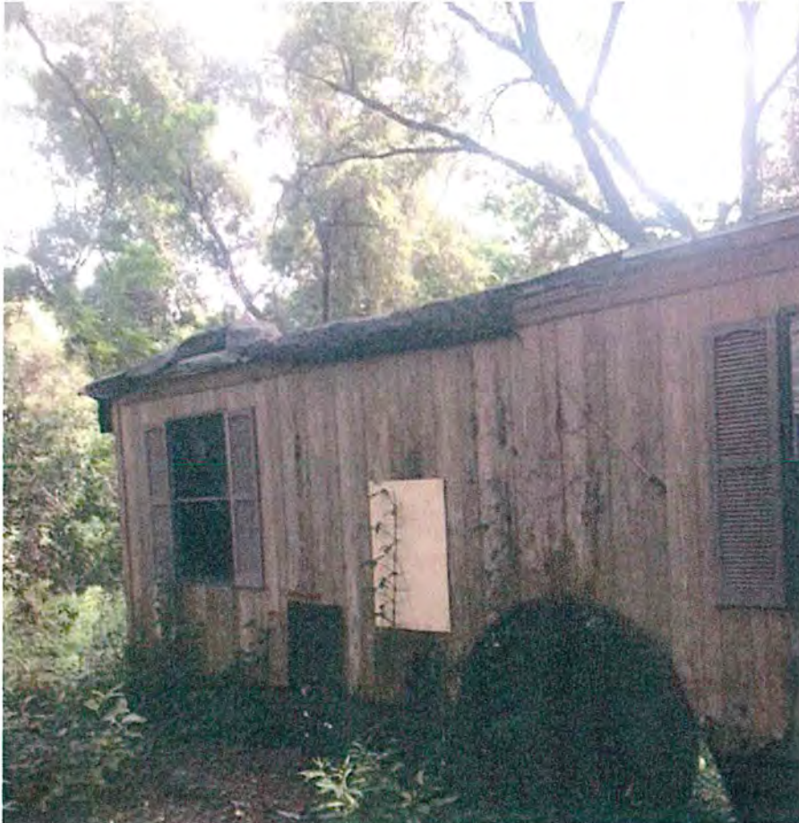
LEFT & SOUTH SIDE VIEW OF MOBILE HOME: WALL PATCHES
