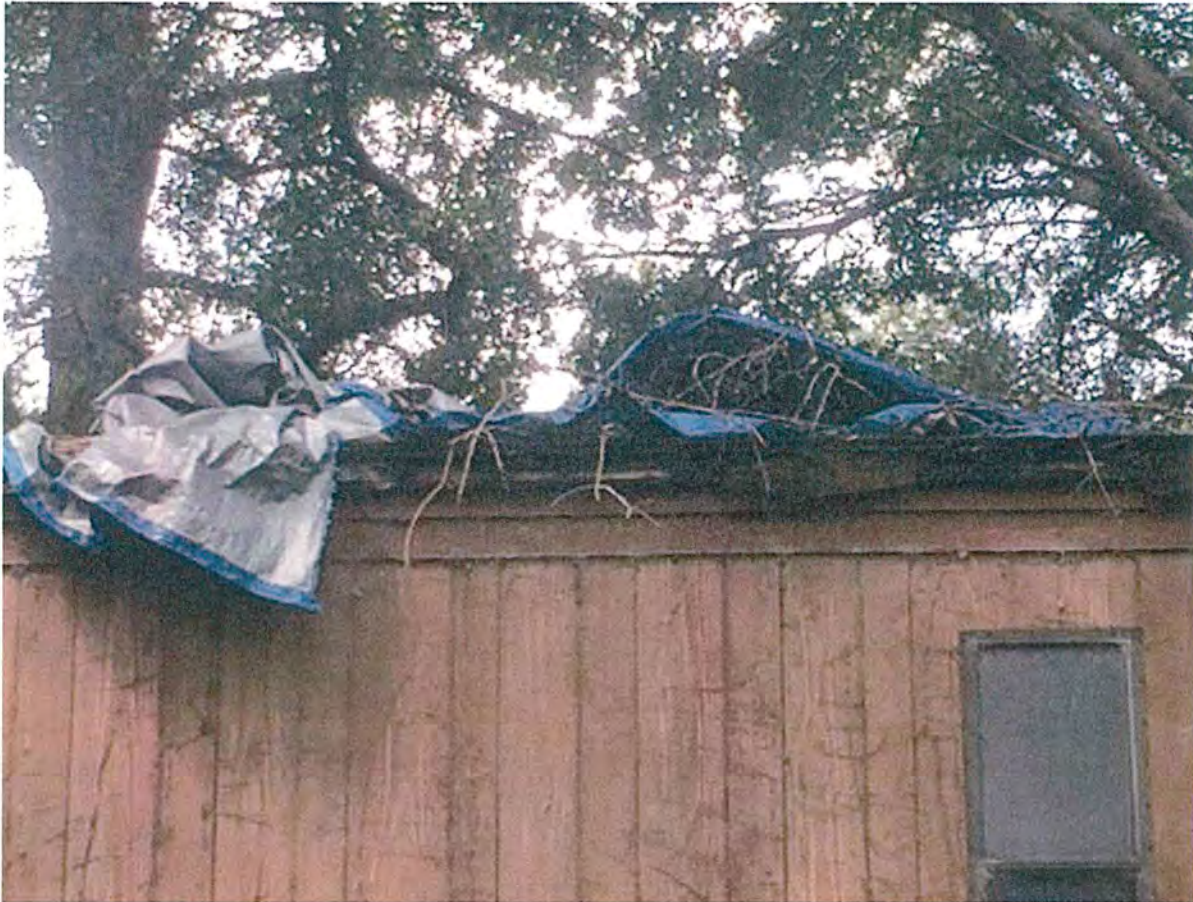
RIGHT & NORTH SIDE VIEW OF MOBILE HOME: LAYERS OF TARPS COVERING ROOF DAMAGE
