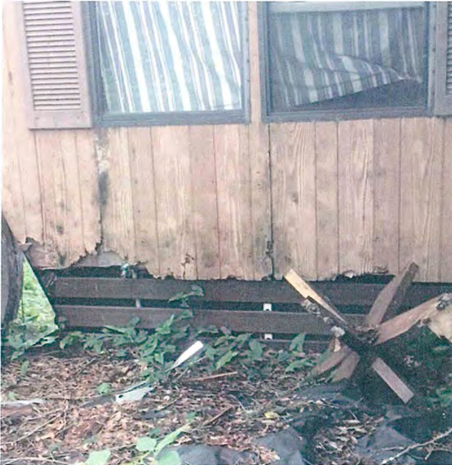
LEFT & SOUTH SIDE VIEW OF MOBILE HOME: WALL ROT & DECAY
