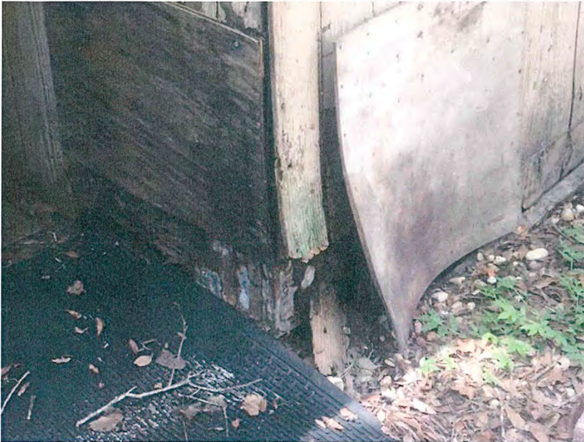
FRONT VIEW OF MOBILE HOME: SOUTH EAST CORNER ROT & DECAY
