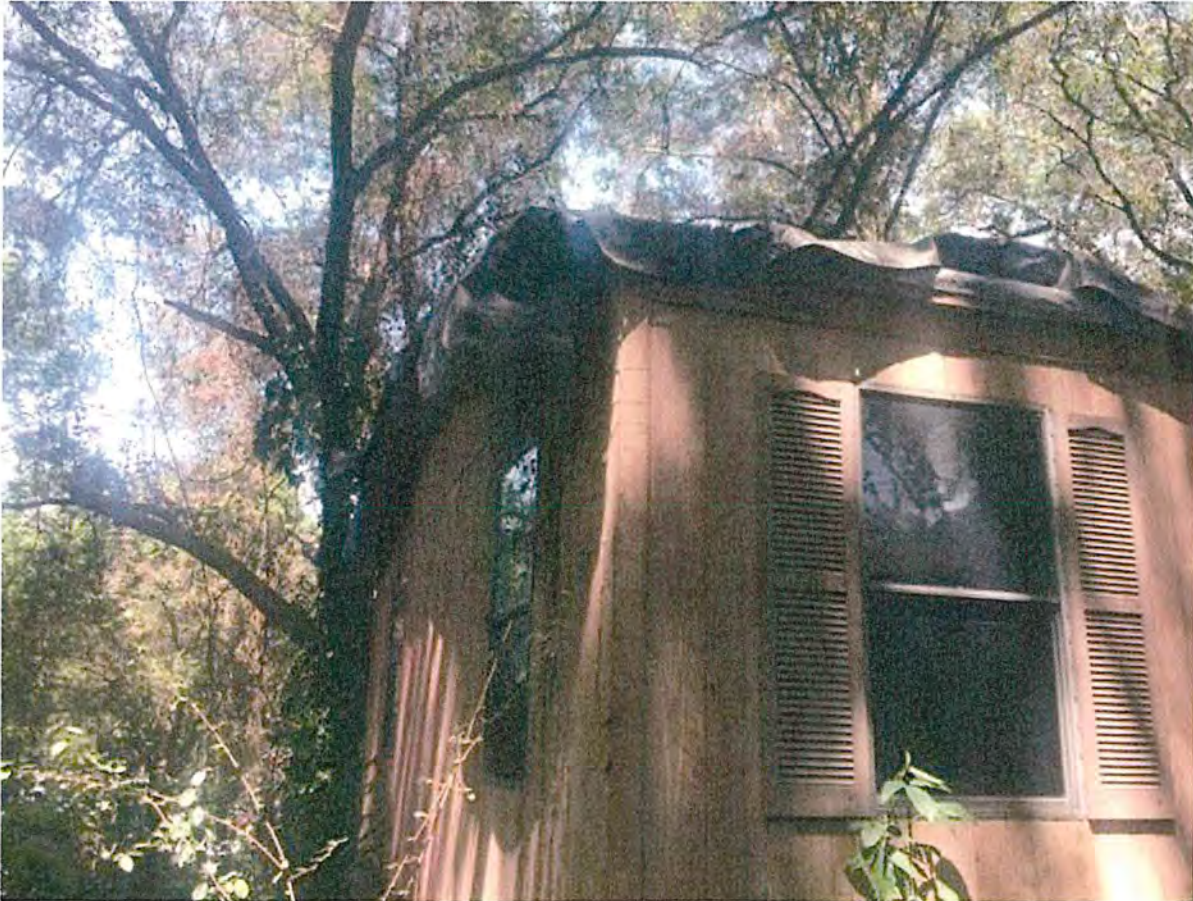
REAR & EAST SIDE VIEW OF MOBILE HOME: ROOF COVERED WITH LAYERS OF TARPS
