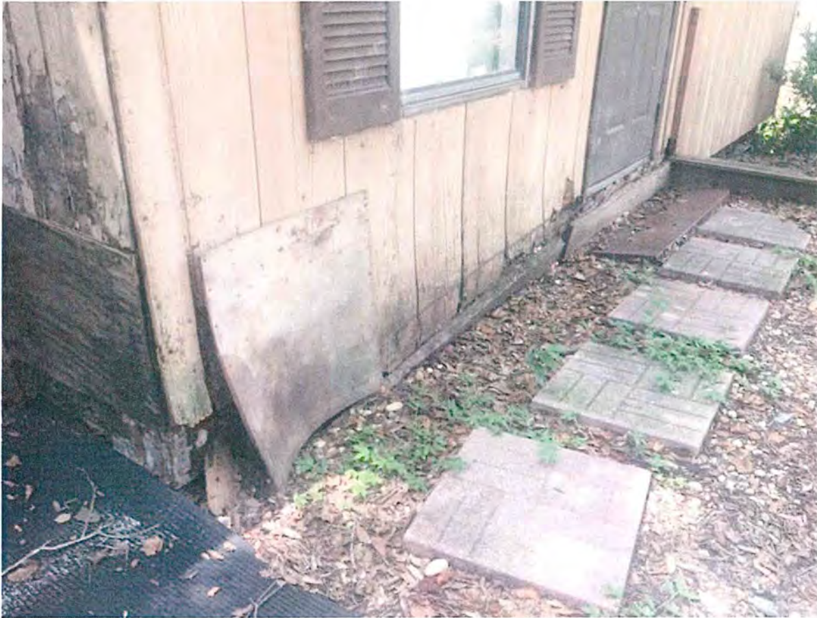
FRONT VIEW OF MOBILE HOME: LOWER WALL AND SIDING ROT & DECAY
