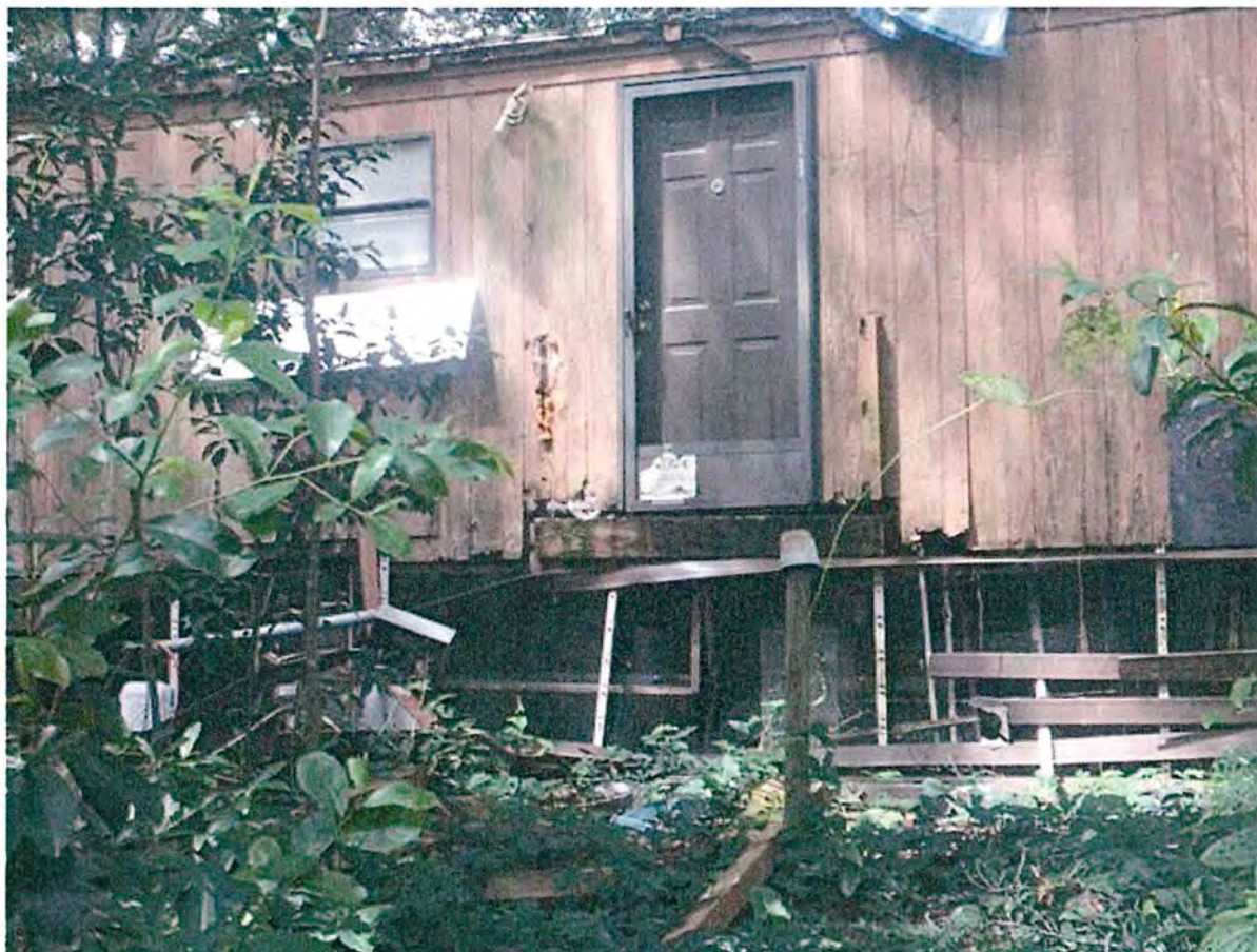
RIGHT & NORTH SIDE VIEW OF MOBILE HOME: SIDE DOOR EXIT DAMAGE & ROT
