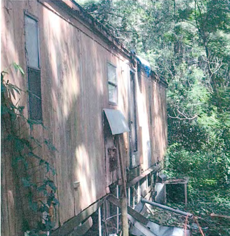
RIGHT & NORTH SIDE VIEW OF MOBILE HOME: DAMAGED SKIRTING
