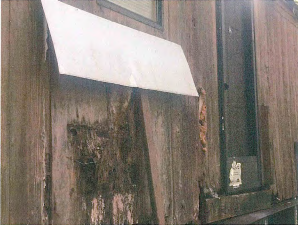
RIGHT & NORTH SIDE VIEW OF MOBILE HOME: WALL ROT & DECAY
