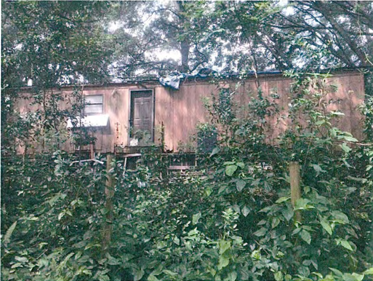
RIGHT & NORTH SIDE VIEW OF MOBILE HOME: ROT & DECAY
