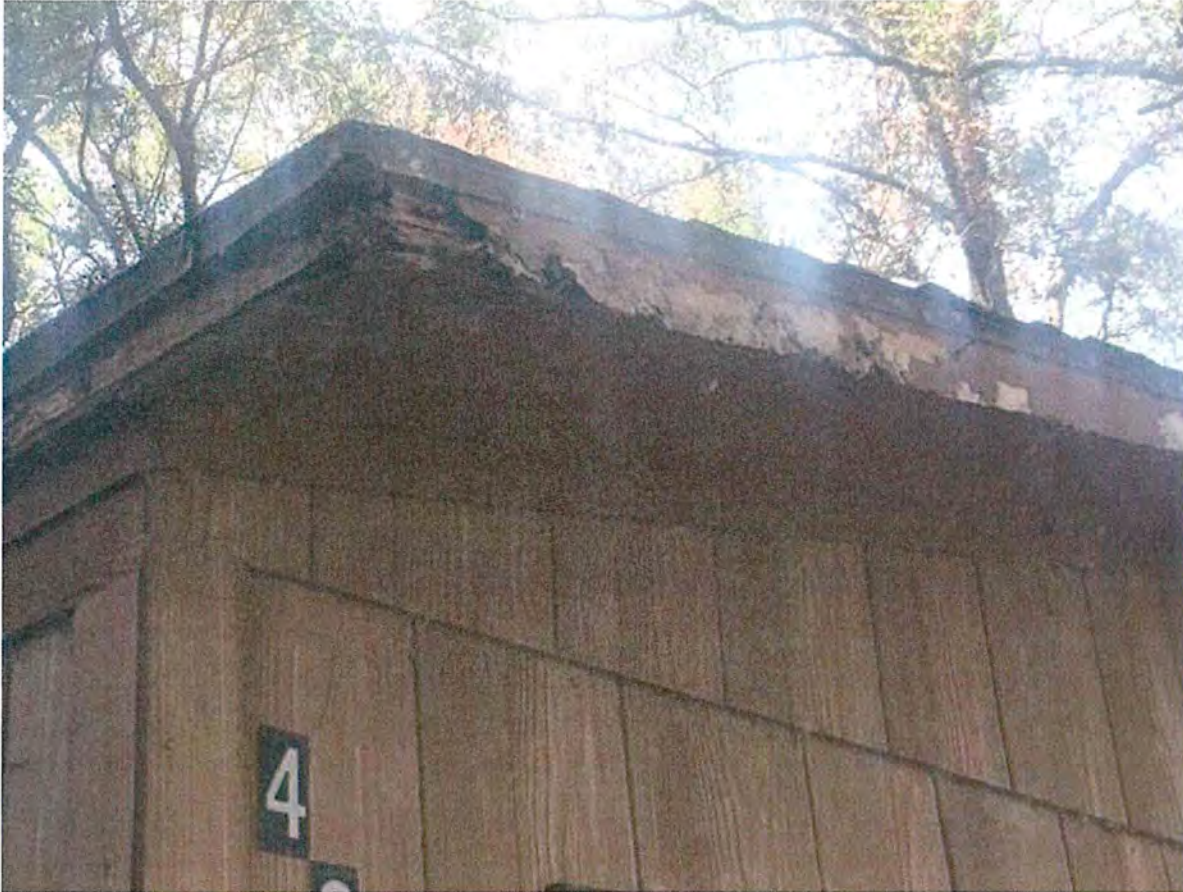
FRONT VIEW OF MOBILE HOME: ROOF ROT & DECAY
