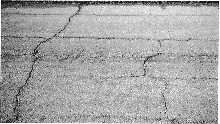
▼ Block cracking with open cracks.
