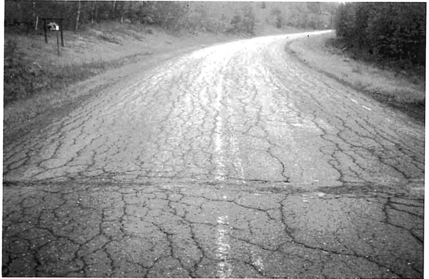
▶ Extensive alligator cracking. Pulverize and rebuild.
