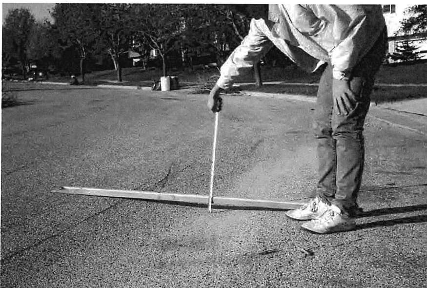
► Severe settling from utility trench.
