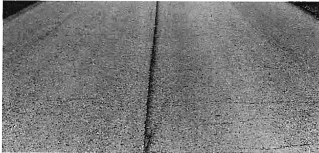
Centerline crack (still tight). ▶
