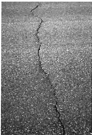
▲ Tight cracks less than 1/4" in width.
