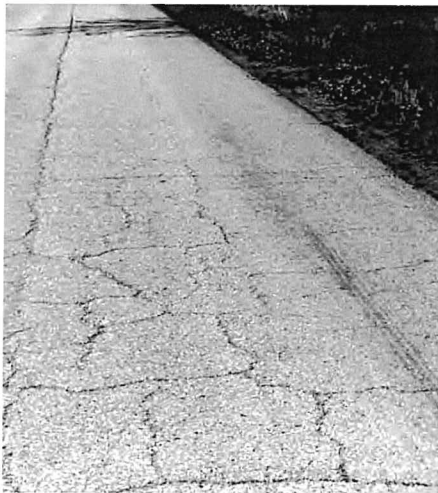
▲ Extensive block cracking in an irregular pattern.
