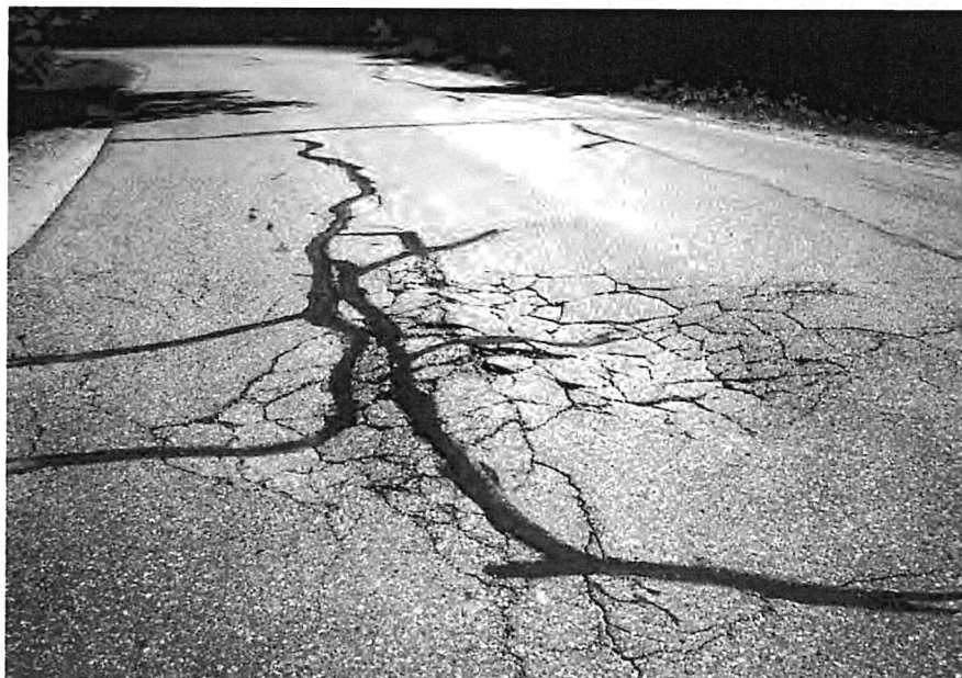
► Frost heave damage from spring break-up.
