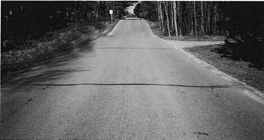
▼ Widely spaced, well-sealed cracks.
