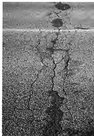
▲ Water enters unsealed cracks softening pavement and causing secondary cracks.
