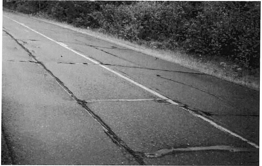
► Concrete joints reflected through bituminous overlay.
