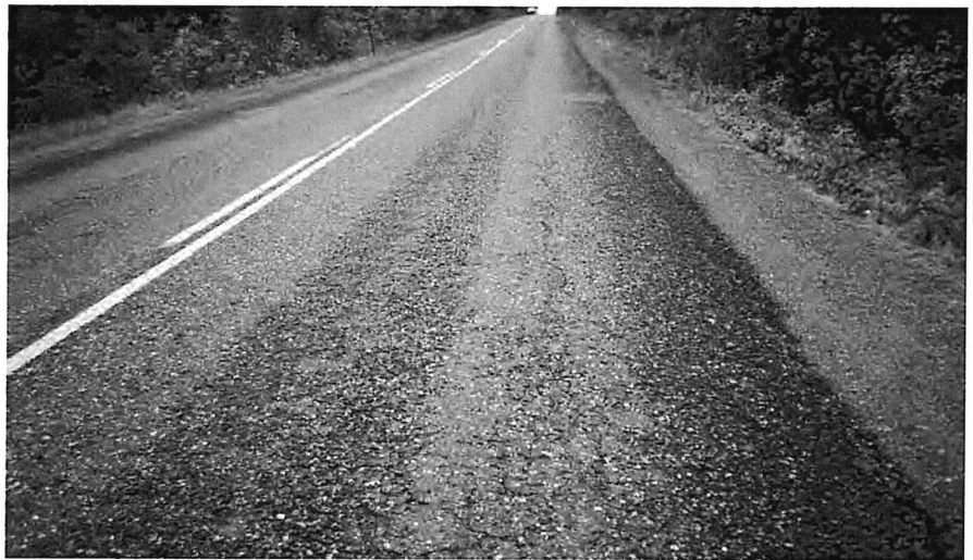
► Moderate to severe raveling in wheel paths.
