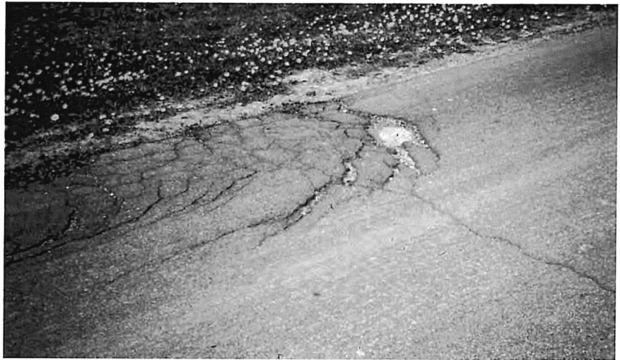
► Crescent-shaped cracks characteristic of slippage.
