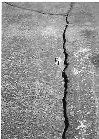
▲ Open crack – 1/2" or more in width.
